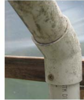
Roof to back wall 45 degree angle PCV pipe joint
