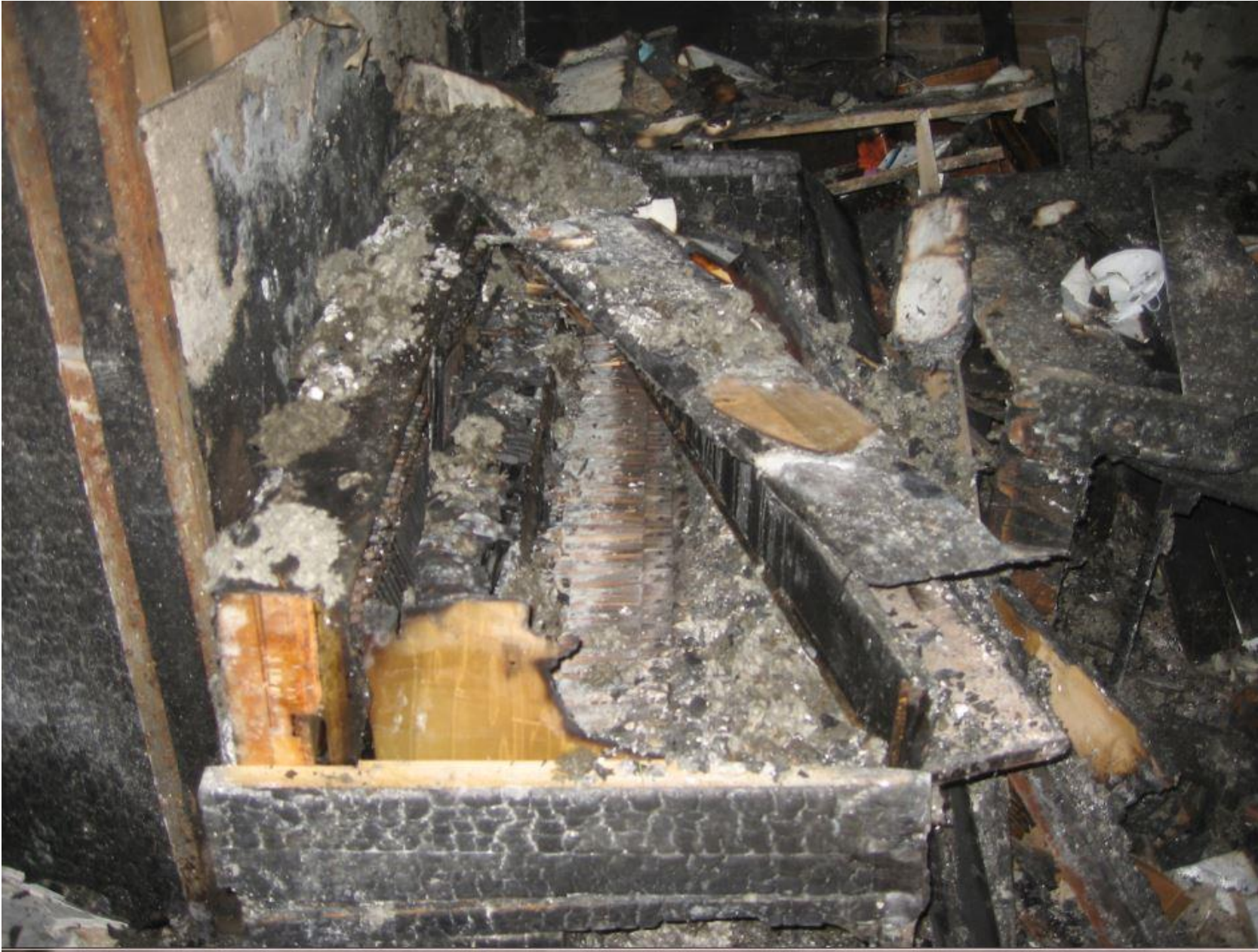
This was a very hot fire that destroyed all of the contents of the entire house
